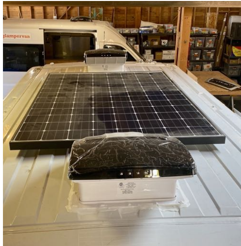
ROOF, NO RACK, MOUNTED SOLAR
